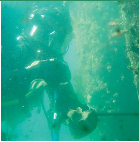
Collins, as a subconsultant to DMJM Harris, provided above and underwater structural inspection and assessment services at Shell's waterfront facility at the Port of Los Angeles. The inspection, performed in accordance with MOTEMS guidelines, was accomplished with a team of four inspectors/divers. Level I, II, and III inspections were conducted to provide an overall condition assessment of the structures, including coring of the timber piles to evaluate the potential deterioration caused by internal marine borers.
