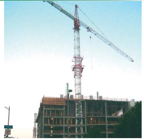
Collins was retained to design a transition detail for a tower crane to be used in the construction of a condominium complex in downtown Los Angeles. The design included steel plate compression and tension checks, bolt and weld design.
