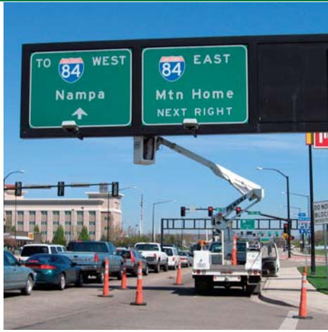
In 2004 and 2005, under separate contracts, Collins was retained by the Idaho Transportation Department to perform field inspections on over 1,000 sign and signal structures located throughout Districts 1, 2, and 3 in the state of Idaho. The different types of structures inspected include sign bridges, cantilever signs, bridge mounted structures, cable spans and signal mast arms.
