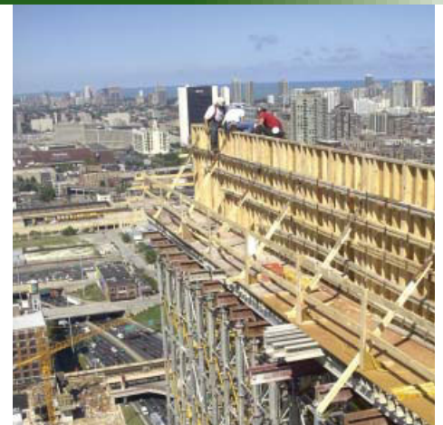
Collins performed steel detailing and scaffolding/formwork design for the architectural appurtenance at the roof of a condominium, a three-story stair tower, and a catwalk between the towers of the building. Collins also provided construction method alternatives for the contractor during construction.
