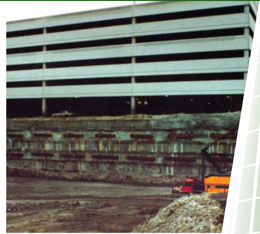
Collins prepared designs and drawings for a tied back soldier pile earth retention system. The excavation was 38 feet deep with one wall approx. 20 feet from an existing parking garage. A concrete facing was used as the excavation was to be open for two years. Collins also performed all proof and performance testing to PTI requirements.
