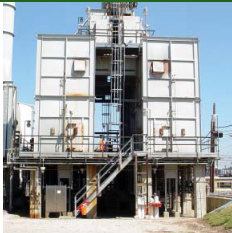
Collins was retained by Marathon Ashland Petroleum to inspect and review the main structural support steel for five coke drums and four platforms to determine the extent of the deterioration of the steel and to determine the existing load carrying capacity of the steel.
